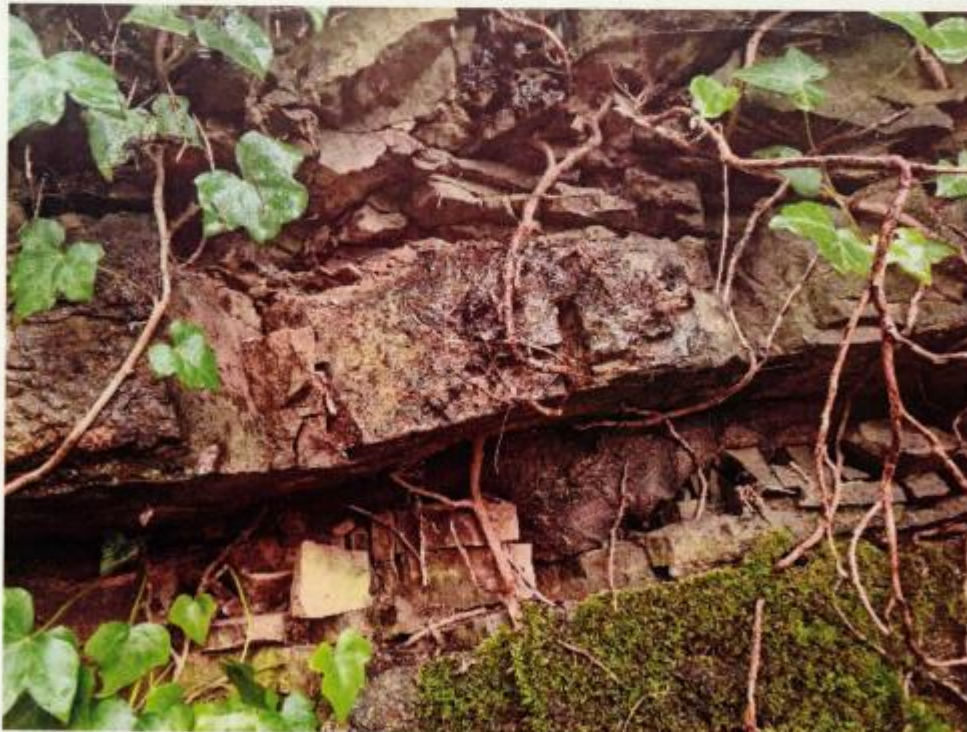
Figure 10: Root penetration, weathering and fracture increase at the slope crest
